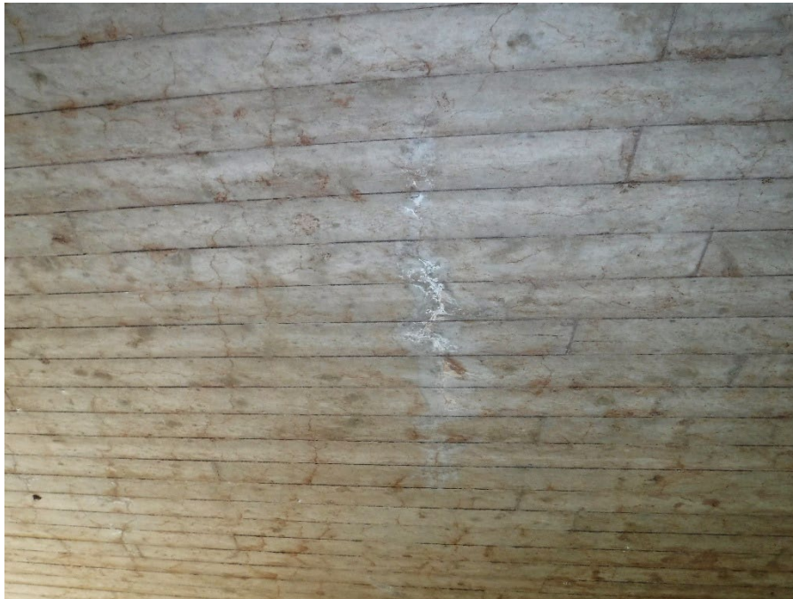
PHOTO 18 LONGITUDINAL CRACK WITH SURFACE WHITE EFFLORESCENCE (10SF 1120 CS2) ON SLAB SOFFIT
