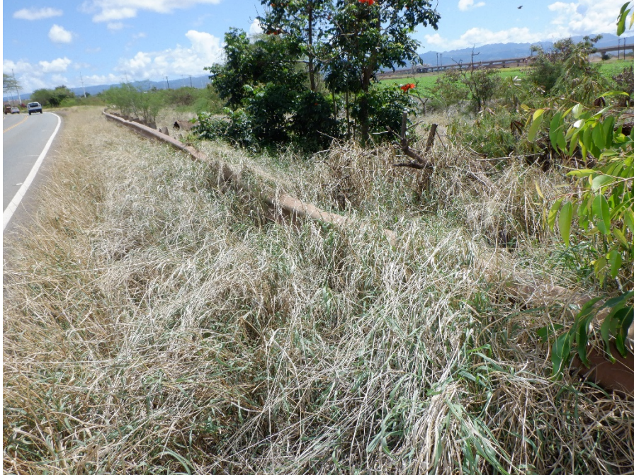
PHOTO 9 HEAVY VEGETATION AT DOWNSTREAM EAST APPROACH GUARDRAIL
