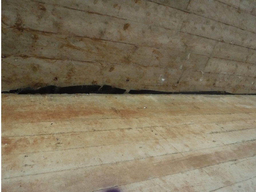
PHOTO 19 PROTRUDING ROOFING PAPER ALONG TOP OF ABUTMENT 1
