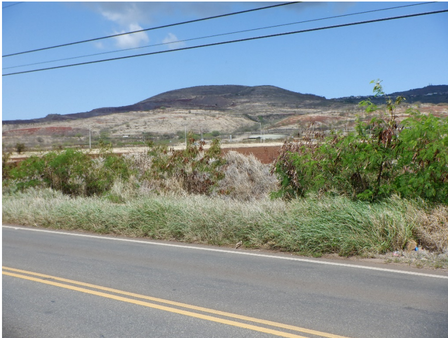
PHOTO 8 UPSTREAM WEST APPROACH GUARDRAIL COVERED BY HEAVY VEGETATION
