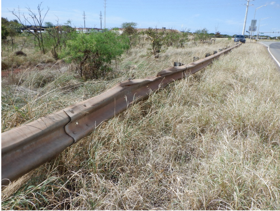
PHOTO 11 IMPACT DAMAGE AT DOWNSTREAM WEST APPROACH GUARDRAIL
