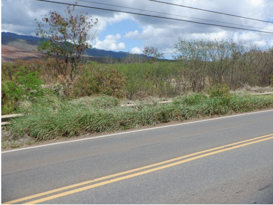
PHOTO 7 HEAVY VEGETATION AT UPSTREAM EAST APPROACH GUARDRAIL
