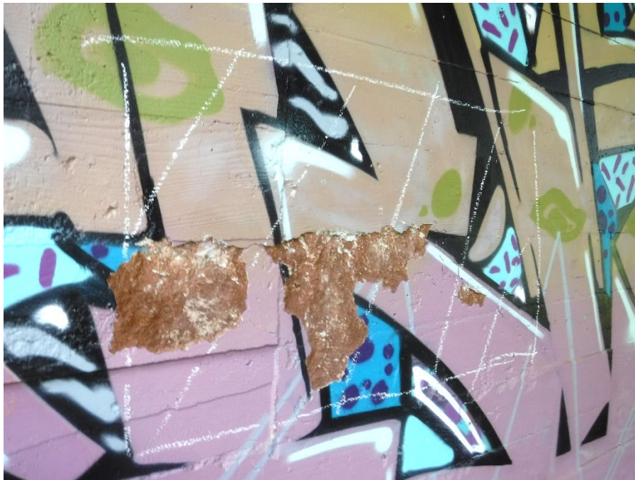
PHOTO 22 3'X2' DELAMINATION (3FT 1080 CS2) ON ABUTMENT 1
