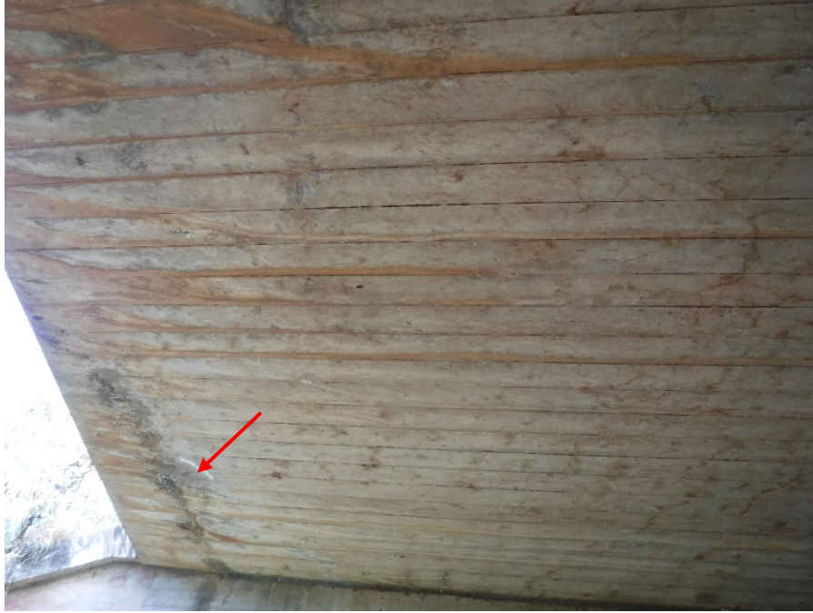
PHOTO 17 8'X1' DELAMINATION (8SF 1080 CS2) AT UPSTREAM EDGE OF SLAB SOFFIT, ADJACENT TO ABUTMENT 2
