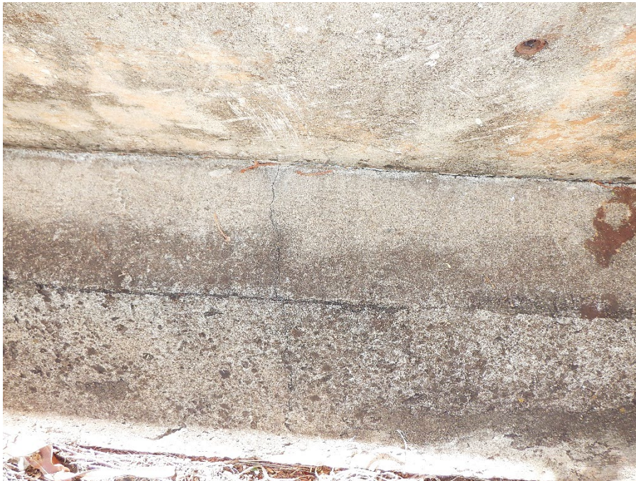
PHOTO 12 TYPICAL TRANSVERSE CRACK ON DOWNSTREAM CURB
