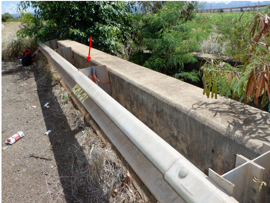
PHOTO 14 TYPICAL IMPACT DAMAGE AT DOWNSTREAM GUARDRAIL POSTS (SEE PHOTO 15)
