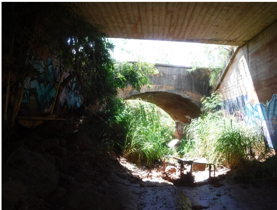
PHOTO 26 DOWNSTREAM CHANNEL WITH HEAVY VEGETATION
