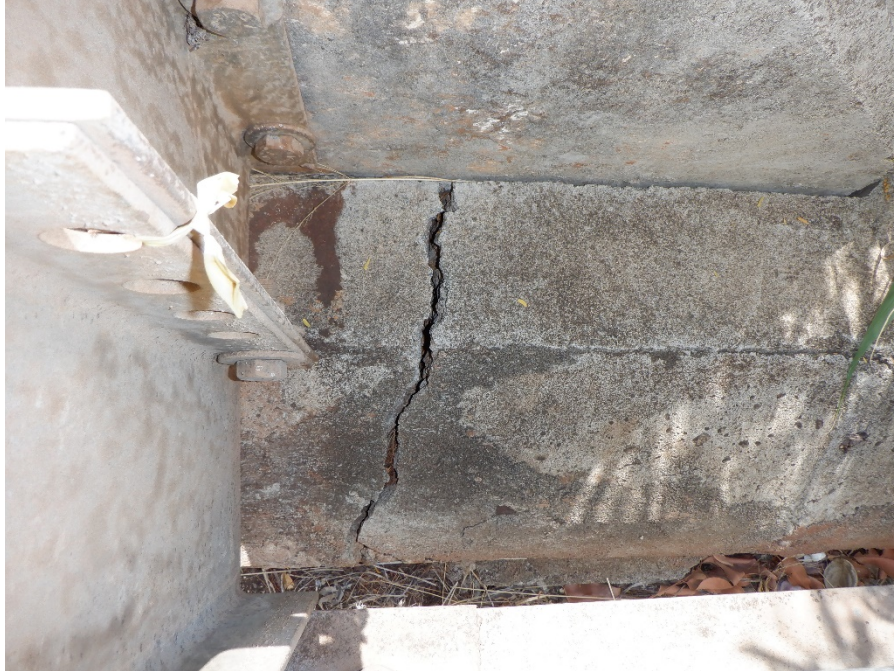
PHOTO 13 1/2" WIDE TRANSVERSE CRACK ON DOWNSTREAM CURB, AT WEST END
