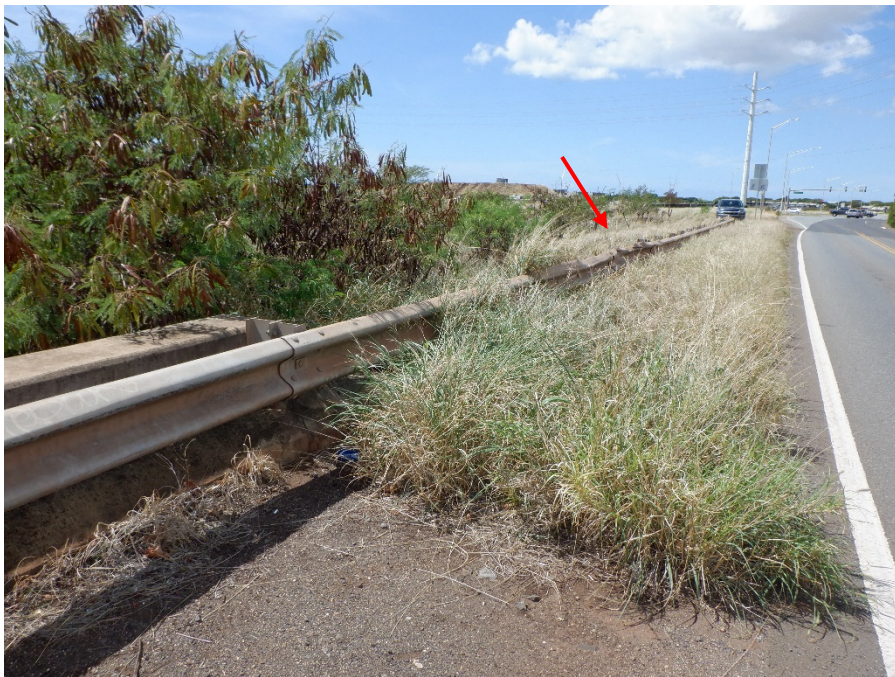
PHOTO 10 DOWNSTREAM WEST APPROACH GUARDRAIL WITH VEGETATION AND IMPACT DAMAGE (SEE PHOTO 11)
