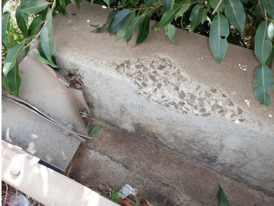
PHOTO 15 1'-6"X6" SPALL (2FT 1080 CS2) ON DOWNSTREAM CONCRETE BRIDGE RAILING AT EAST END OF BRIDGE AND IMPACT DAMAGE AT GUARDRAIL POST
