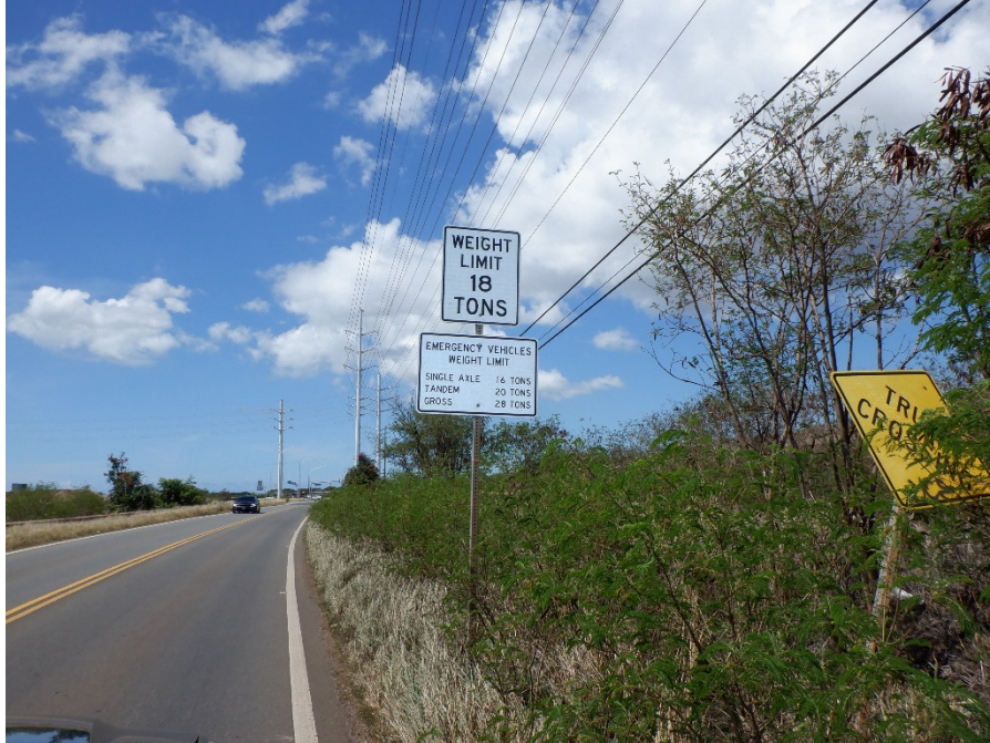
PHOTO 5 LOAD POSTING SIGNS AND BENT TRUCK CROSSING SIGN ON FARRINGTON HIGHWAY AT EAST APPROACH TO BRIDGE
