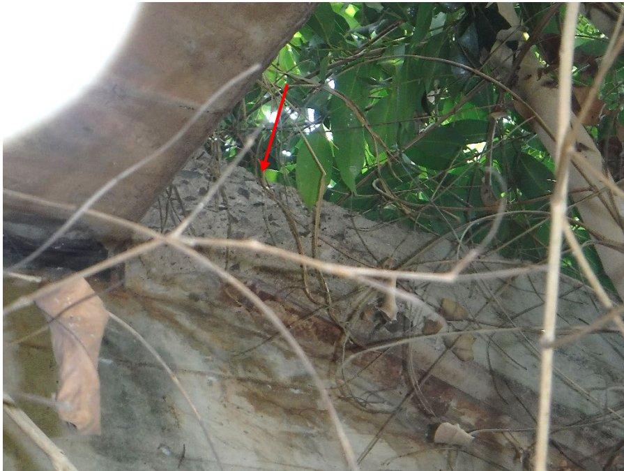
PHOTO 24 2'X1' SPALL AT TOP OF DOWNSTREAM EAST WINGWALL
